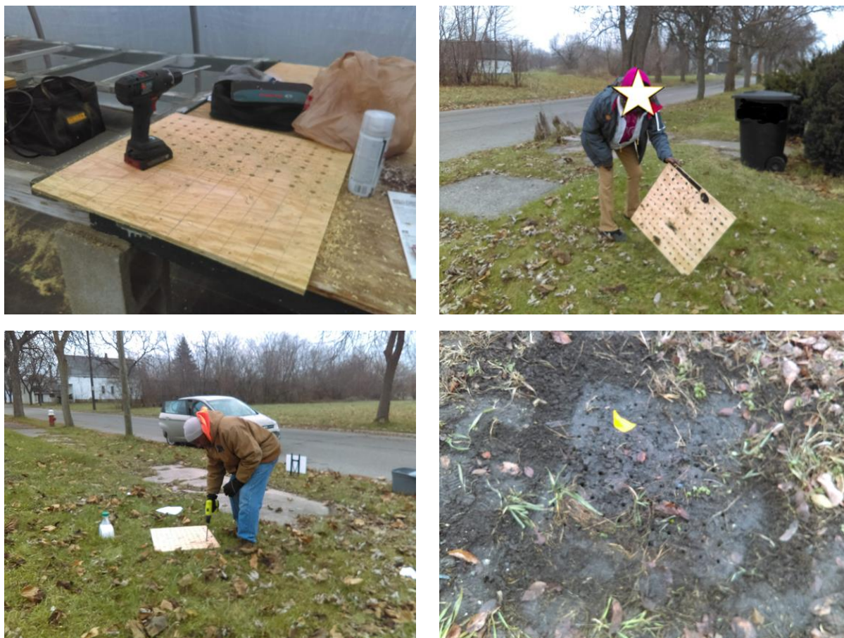
Figure 5.2. Construction of amendment application apparatus and resulting holes in soil where bone meal solution is applied.
