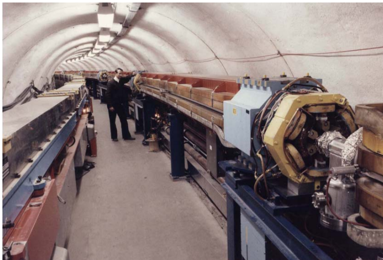
Figure 2.2: Picture taken in the tunnel, with synchrotron on the left and storage ring on the right
